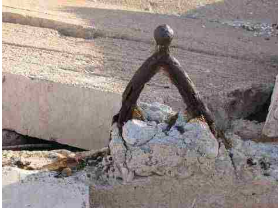
Figure 18: Front suspension piece from an old automobile used as concrete reinforcement, Hannig's Ice Cream Parlor. Photo by author.
