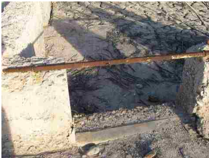
Figure 19: Axle used as concrete/window frame reinforcement, Samuel Gentry home. Photo by author.
