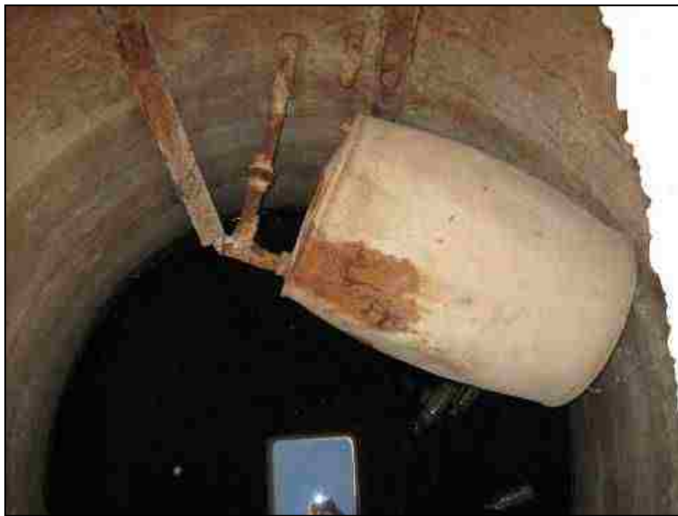
Figure 28: Plumbing in the school's cistern, February 2008. Photo by author.
